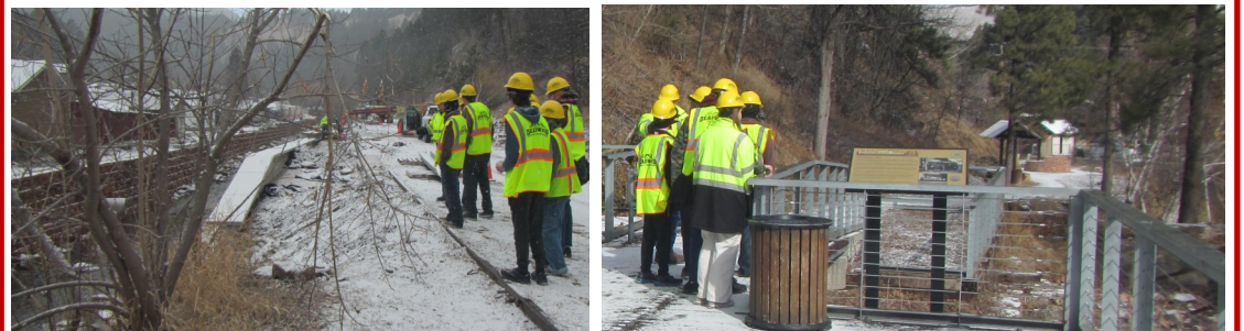
Pictured above: Students tour the FEMA worksite along Whitewood Creek. They learned about the damage that was caused by flooding in 2019 and how FEMA is paying for repairs and improvements to the creek and surrounding areas.
