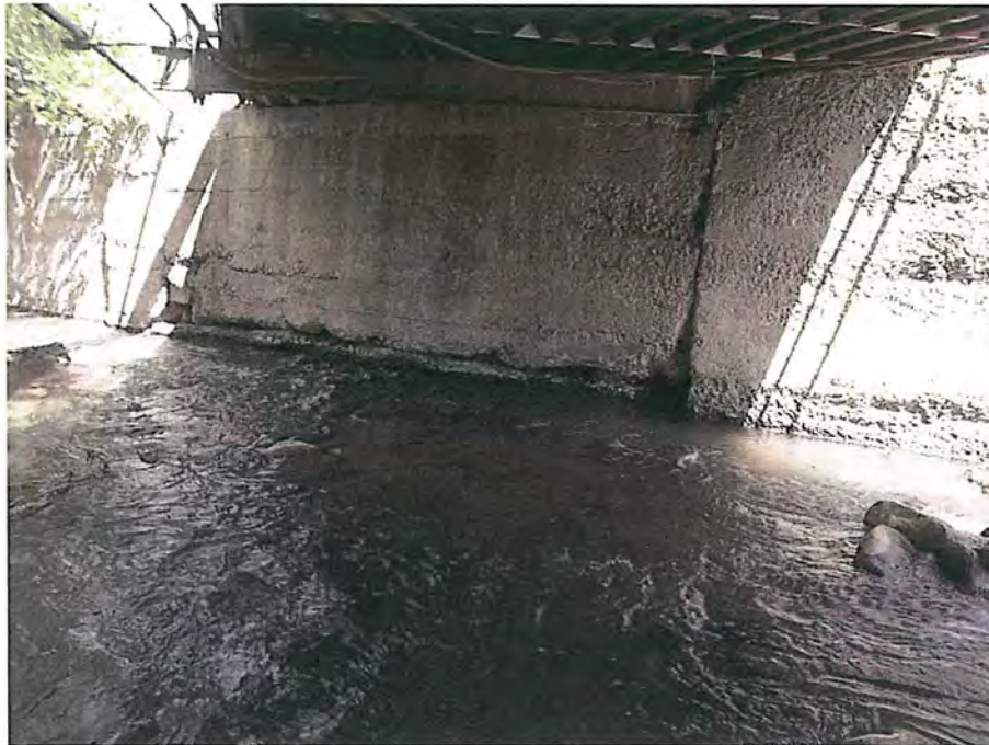
View of deterioration of East abutment City of Deadwood, Charles Street Bridge 31.JPG 5/25/2016
