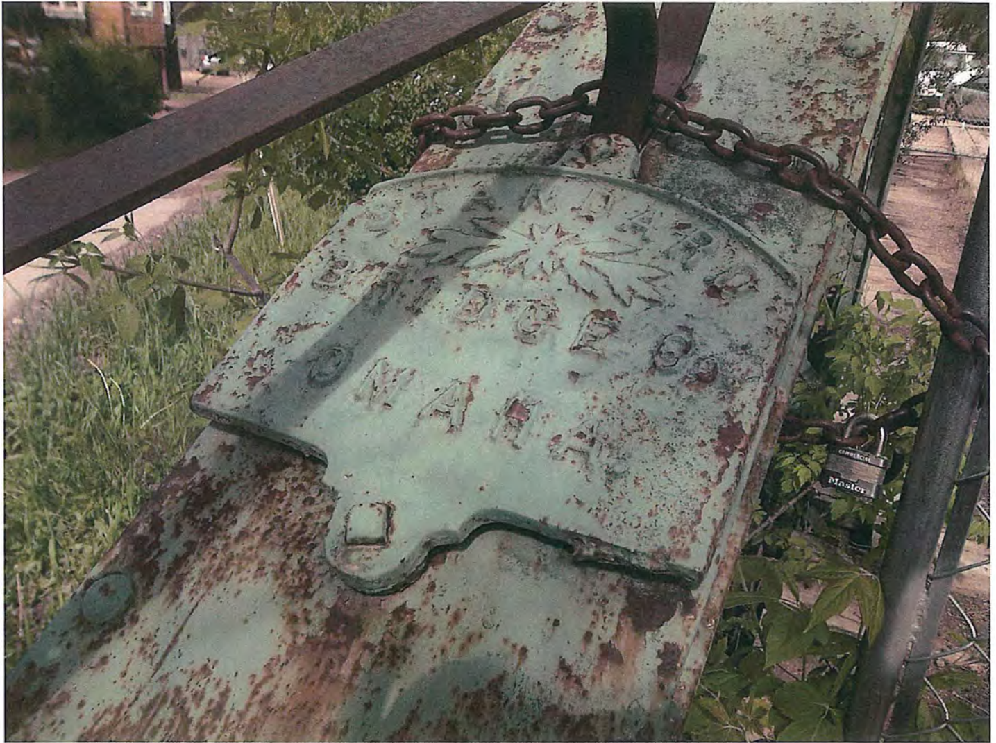
Manufacturers bolt on name plate City of Deadwood, Charles Street Bridge 37.JPG 5/25/2016
