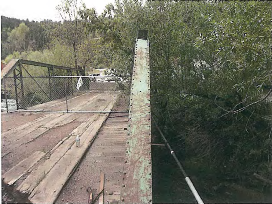
Northeast corner of the truss in leaning outward City of Deadwood, Charles Street Bridge 5.JPG 5/25/2016
