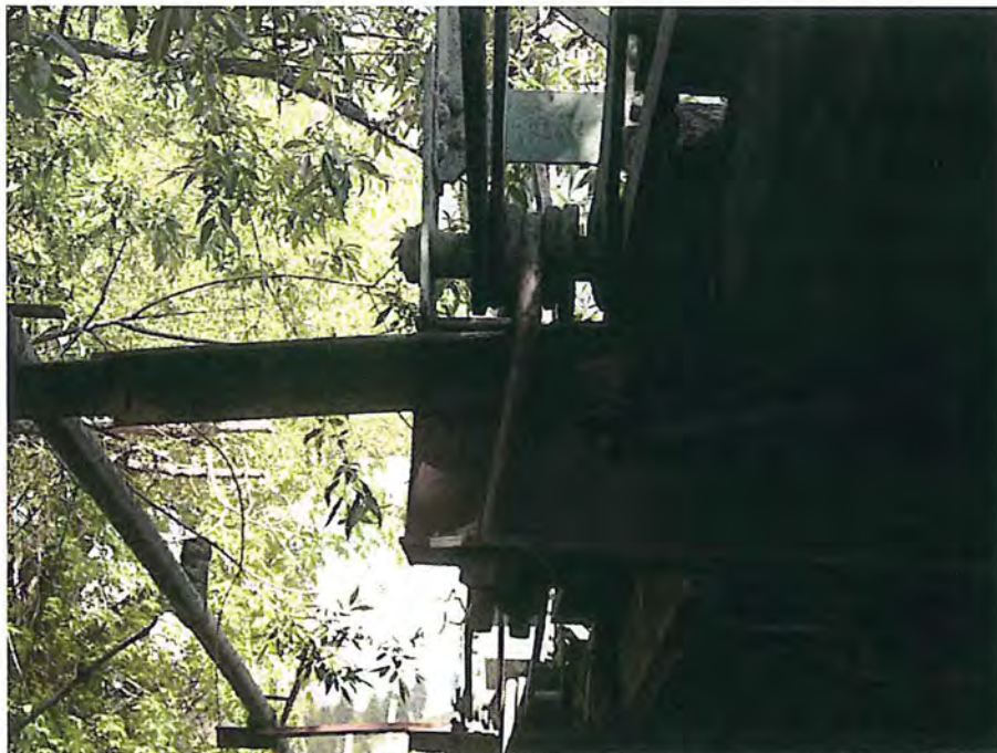
Bent floor beam hanger on the North side of the structure City of Deadwood, Charles Street Bridge 35.JPG 5/25/2016
