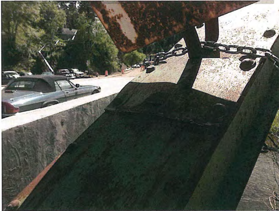
Pack rust on splice in diagonal member at Southeast corner (top) City of Deadwood, Charles Street Bridge 22.JPG 5/25/2016
