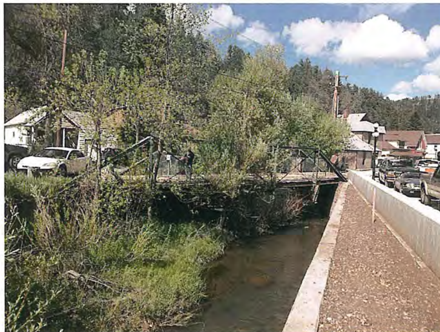
View of the South bridge opening City of Deadwood, Charles Street Bridge 36.JPG 5/25/2016
