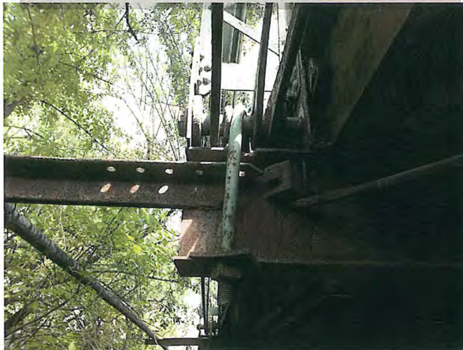
Connection of hanging floor beam to the pin of the lower cord (typical) City of Deadwood, Charles Street Bridge 27.JPG 5/25/2016
