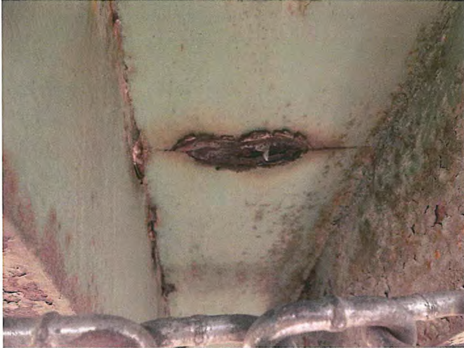
Pack rust on splice in diagonal member at Southeast corner (bottom) City of Deadwood, Charles Street Bridge 21.JPG 5/25/2016
