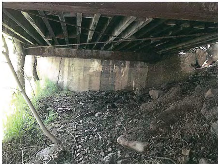
View of the West abutment with the North end of the West floor beam encased in concrete City of Deadwood, Charles Street Bridge 32.JPG 5/25/2016
