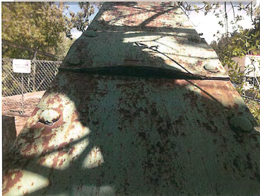
Pack rust on splice in diagonal member at Northwest corner (top) City of Deadwood, Charles Street Bridge 19.JPG 5/25/2016
