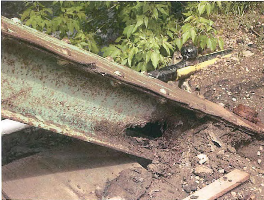
Hole through web of member at Northeast corner City of Deadwood, Charles Street Bridge 3.JPG 5/25/2016
