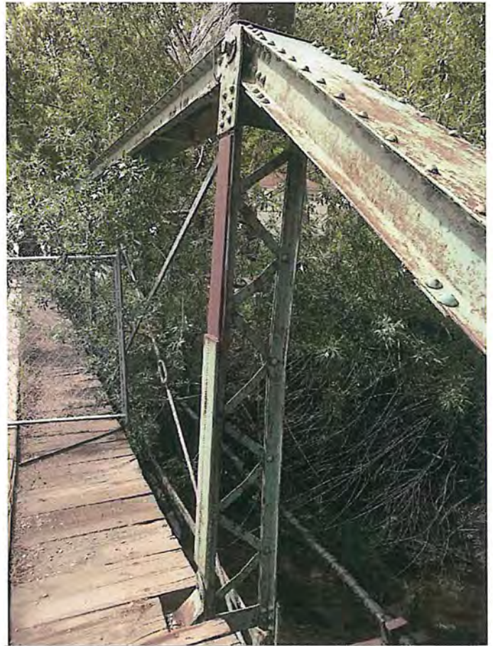
Welded splice on the Northeast vertical member that has been broken (V4) City of Deadwood, Charles Street Bridge 6.JPG 5/25/2016
