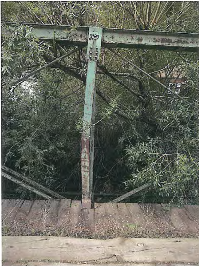
Bent vertical member on South side (V2) City of Deadwood, Charles Street Bridge 9.JPG 5/25/2016
