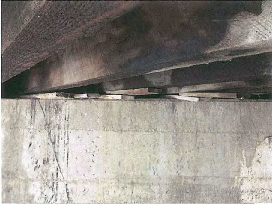
Timber shims under timber stringers on west end of bridge City of Deadwood, Charles Street Bridge 24.JPG 5/25/2016
