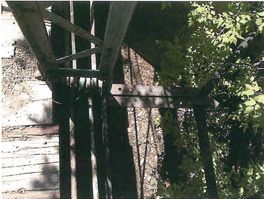
Angle iron supports for suspended gas line on North side of bridge City of Deadwood, Charles Street Bridge 20.JPG 5/25/2016
