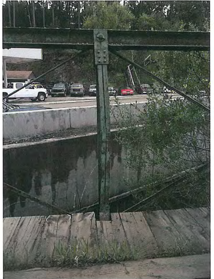
Bent vertical member on South side (V3) City of Deadwood, Charles Street Bridge 15.JPG 5/25/2016
