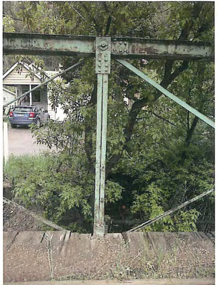
Bent Vertical member on North side (V2) City of Deadwood, Charles Street Bridge 10.JPG 5/25/2016
