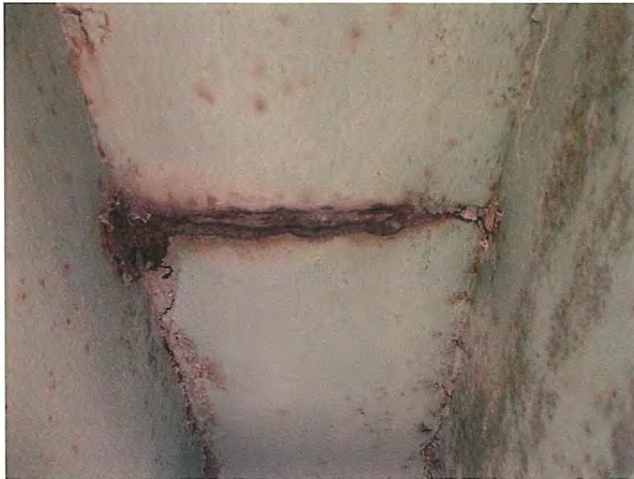
Pack rust on splice in diagonal member at Northwest corner (bottom) City of Deadwood, Charles Street Bridge 18.JPG 5/25/2016
