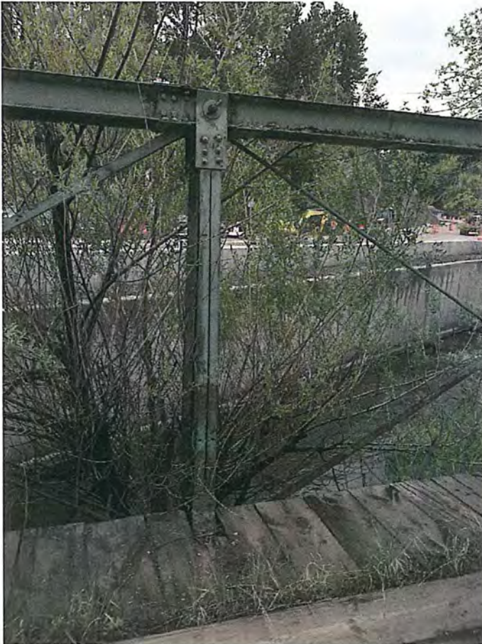
Bent vertical member on South side (V2) City of Deadwood, Charles Street Bridge 14.JPG 5/25/2016
