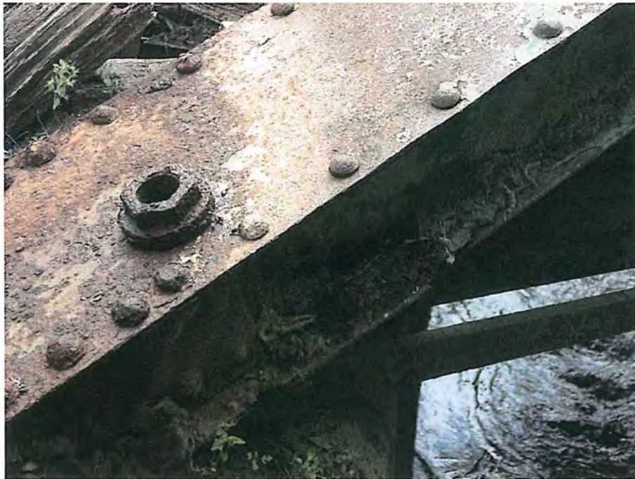
Hole through web of member at Northeast corner City of Deadwood, Charles Street Bridge 4.JPG 5/25/2016
