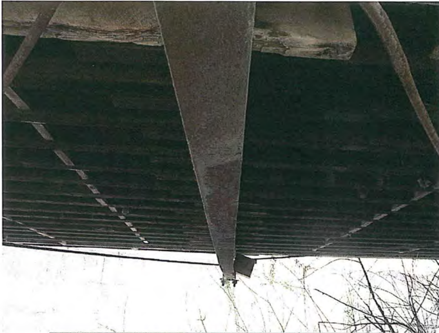
Twisted floor beam near the center of the structure City of Deadwood, Charles Street Bridge 28.JPG 5/25/2016
