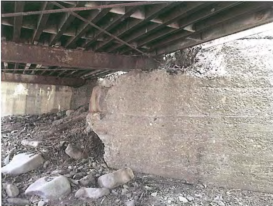
View of the North end of the second floor beam supported by old concrete wall City of Deadwood, Charles Street Bridge 33.JPG 5/25/2016
