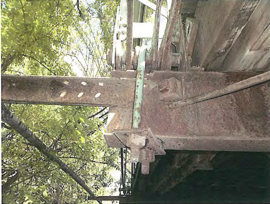
Connection of hanging floor beam to the pin of the lower cord (typical) City of Deadwood, Charles Street Bridge 26.JPG 5/25/2016
