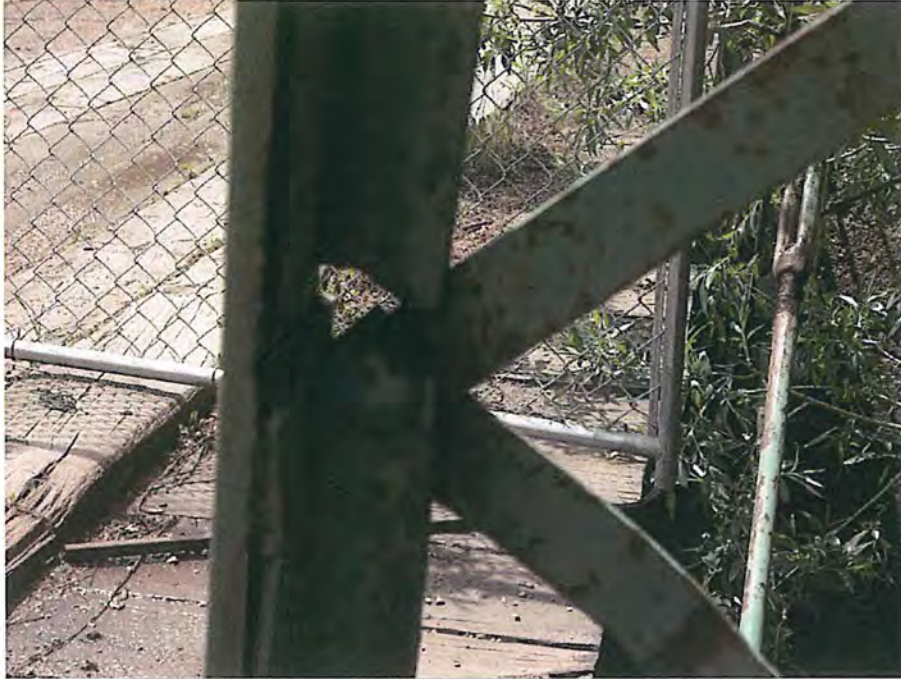
Area of break on North vertical member (V4) City of Deadwood, Charles Street Bridge 7.JPG 5/25/2016
