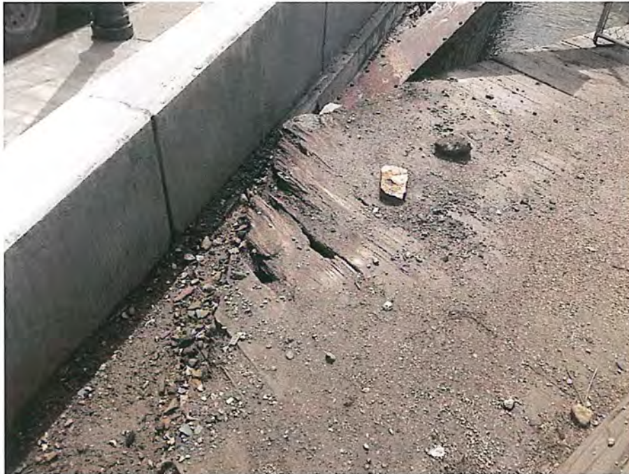
Deterioration of the Southeast corner of the timber deck City of Deadwood, Charles Street Bridge 8.JPG 5/25/2016
