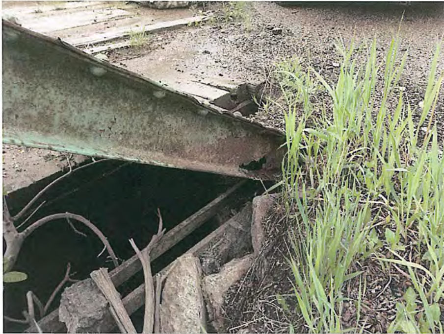
Hole through web of member at Northwest corner City of Deadwood, Charles Street Bridge 12.JPG 5/25/2016
