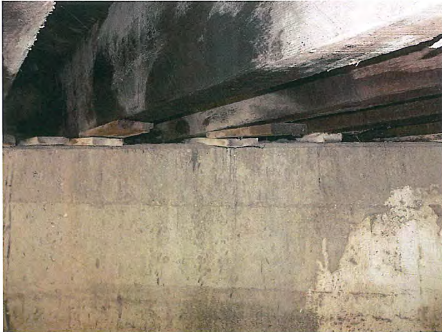
Timber shims under timber stringers on west end of bridge City of Deadwood, Charles Street Bridge 25.JPG 5/25/2016
