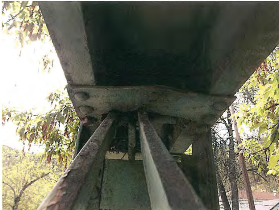
Bent plate on top chord from diagonal members (typical) City of Deadwood, Charles Street Bridge 17.JPG 5/25/2016
