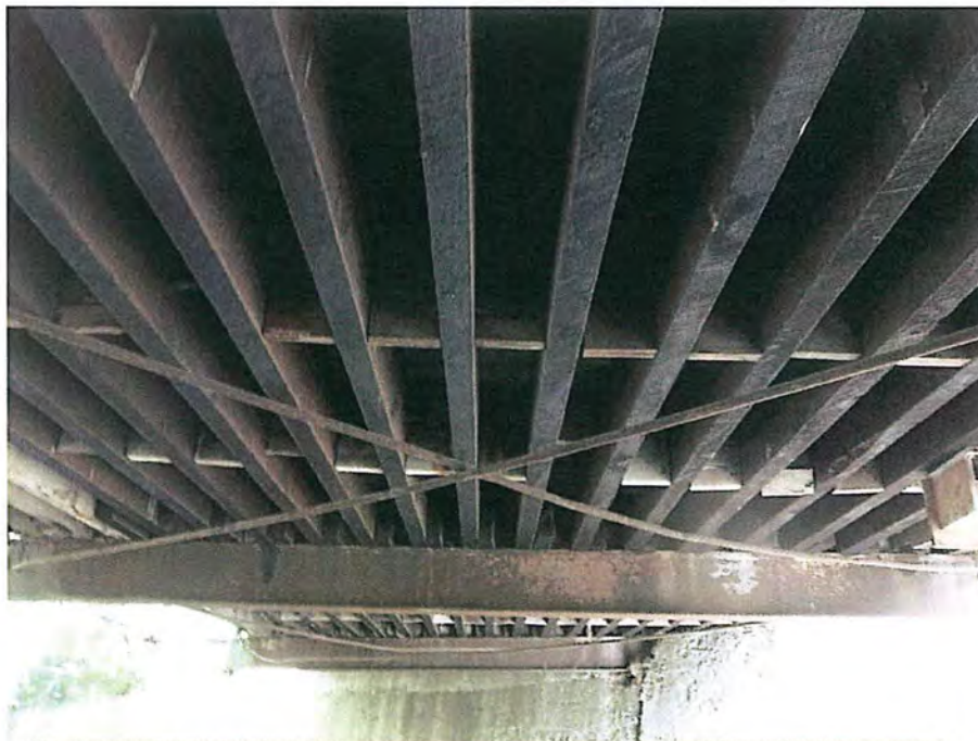
View of the timber stringers and steel floor beams with loose and bent diagonal sway bracing City of Deadwood, Charles Street Bridge 29.JPG 5/25/2016
