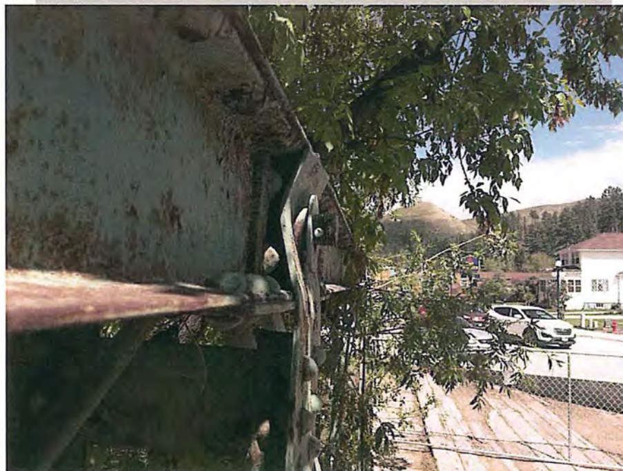
Bent gusset plate connector of vertical member to top cord (typical) City of Deadwood, Charles Street Bridge 23.JPG 5/25/2016
